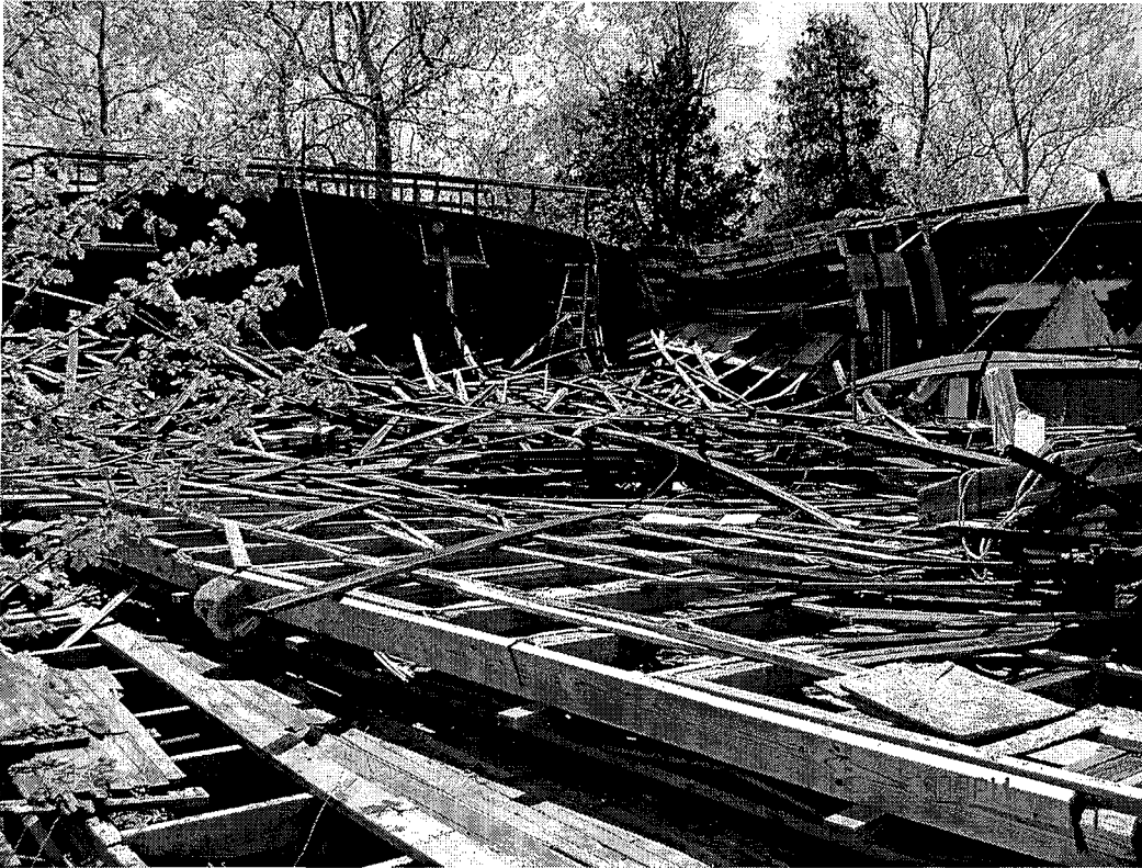
Date: 05/04/2005 Time: 1:09 p.m. Direction: southwest Photo by: Bill Gonet Exposure #: 005 Comments: General const/demo debris.
