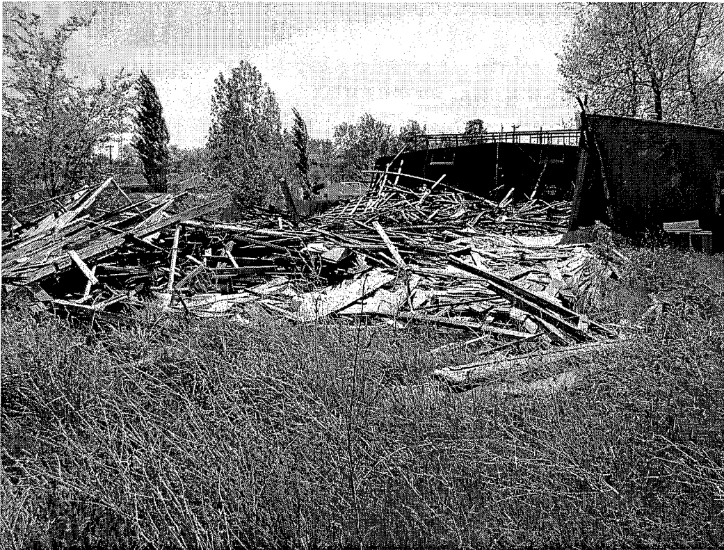
Date: 05/04/2005 Time: 1:08 p.m. Direction: southeast Photo by: Bill Gonet Exposure #: 003 Comments: General const/demo debris.
